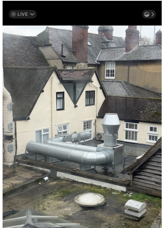
Fig. 6 — Context view of the installed system showing the wider backland area. Multiple existing roof-mounted plant items and AC units are visible on neighbouring properties, demonstrating the established servicing character of this area.
