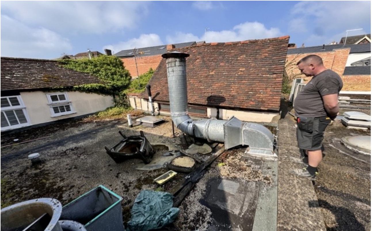
Fig. 3 — Pre-installation condition of the flat roof showing the old, non-compliant extraction system mid-removal. The dilapidated ductwork, corroded components, and general state of disrepair are evident. The new system connects to the same pre-existing roof openings. Source: Fusion Hot Ltd, October 2025.
