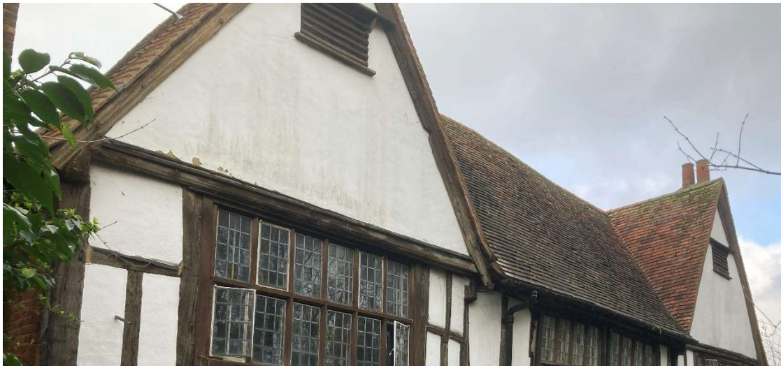
Louvred panels in east facing gables help to ventilate the roof space
