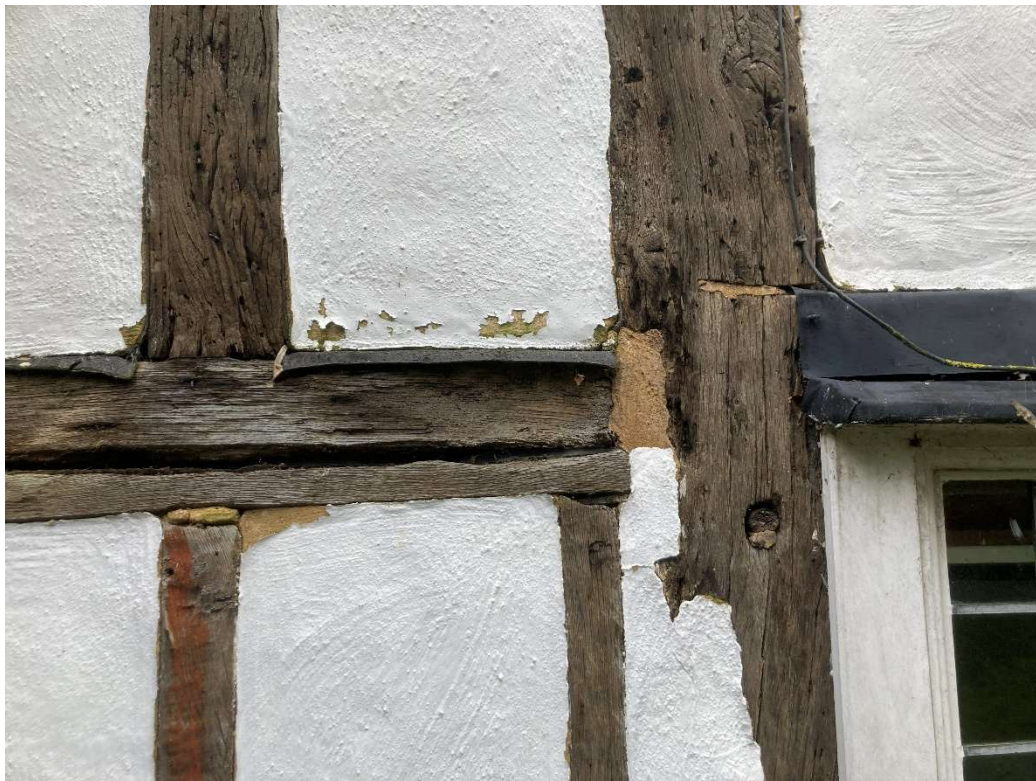
Roofing felt used to flash oak plate/ Peeling paint suggesting the paint finish is not breathable/ Render below the plate seems to have a cementitious base; above the plate the render may have a lime base.
