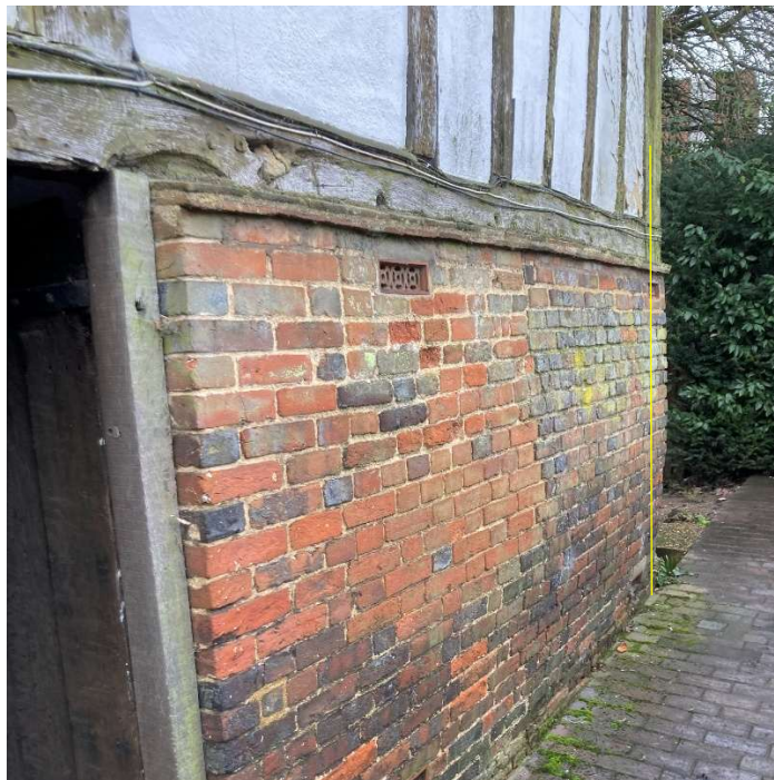
Bowing in the masonry west of the access into the courtyard
