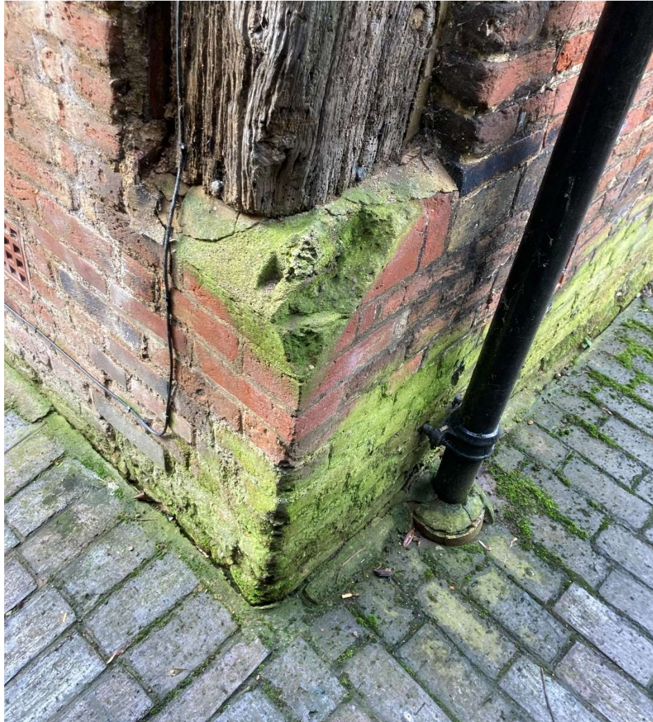
North-east corner post: Note algae/ moss growth indicating consistent dampness in the lower wall
