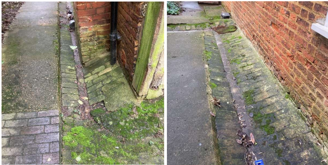
Damp in the base of the south wall caused by the drainage channel
