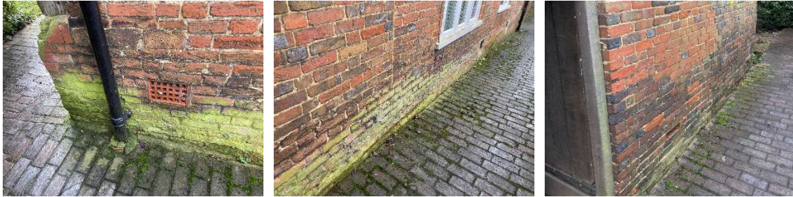
Excessive dampness causing moss and algae growth along the base of the wall
