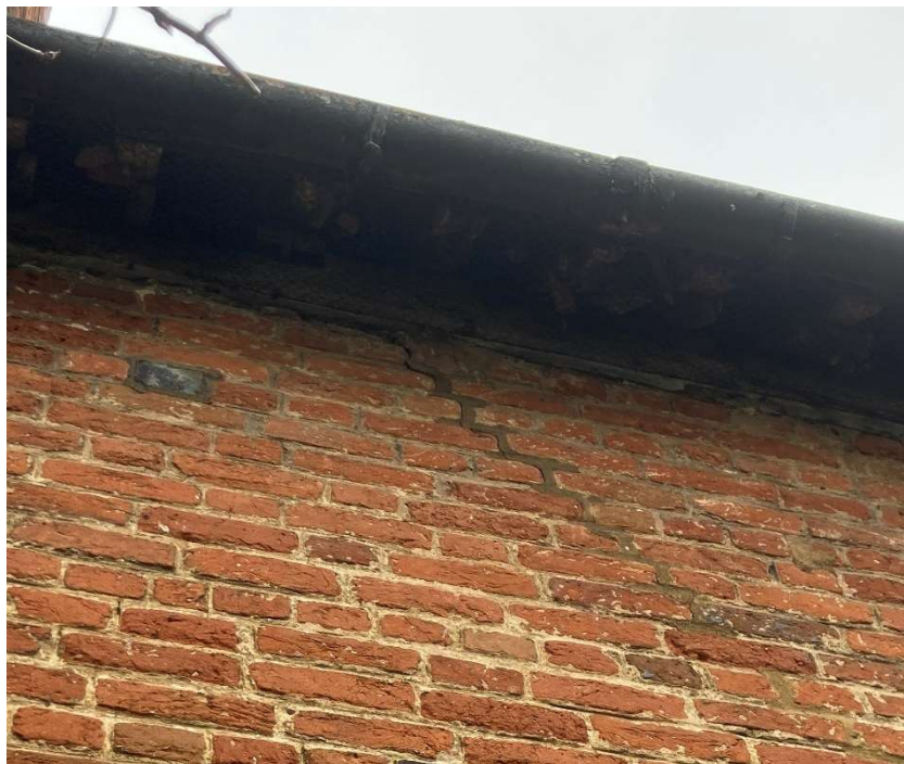
Previously cracked and filled masonry – Further review required
