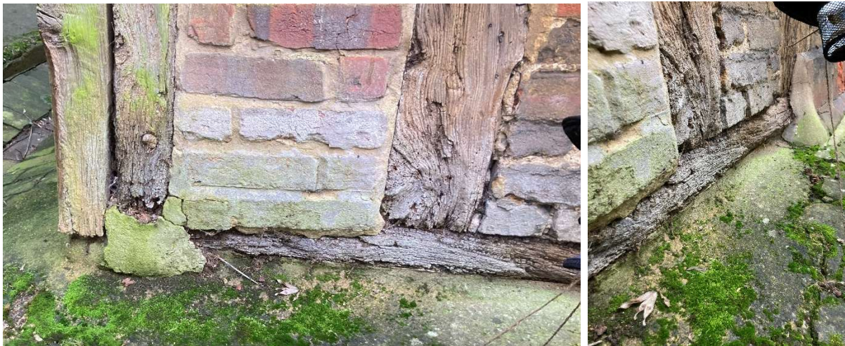
Rot in the south-east corner post, stud bases and sole plate
