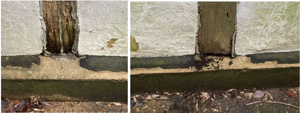
Concrete plinth and decayed stud bases
