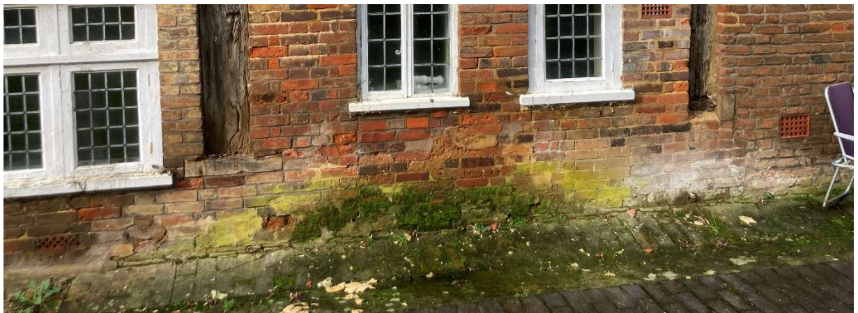
Excessive damp in the base of the eastern elevation and the drainage channel
