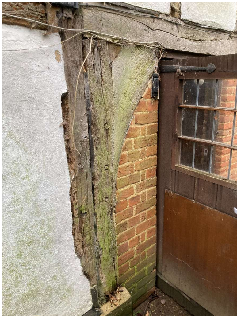
Original post and haunch, severely decayed
