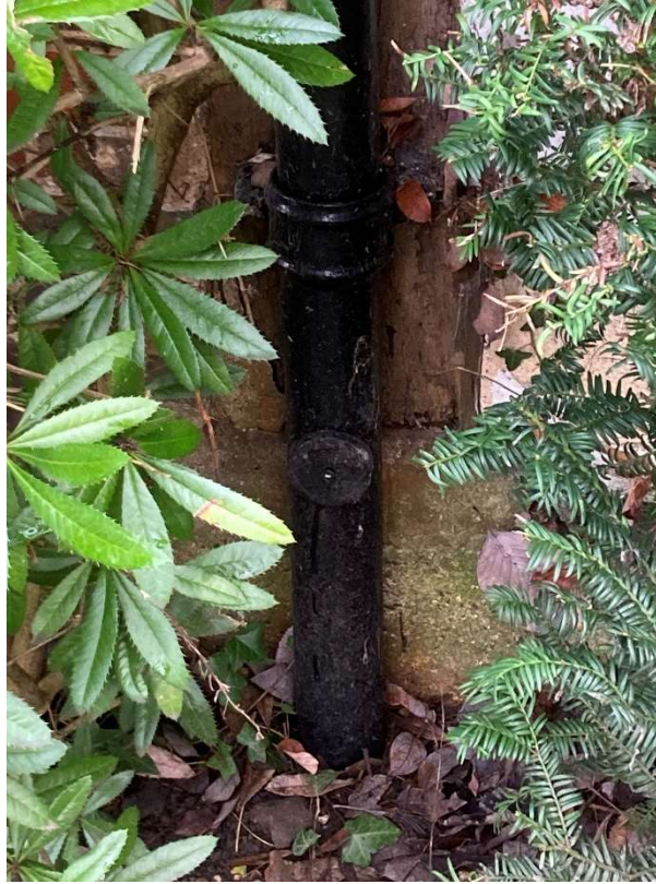
Stud base behind downpipe, partially concealed. Rot in the base of the stud above the concrete skirt.
