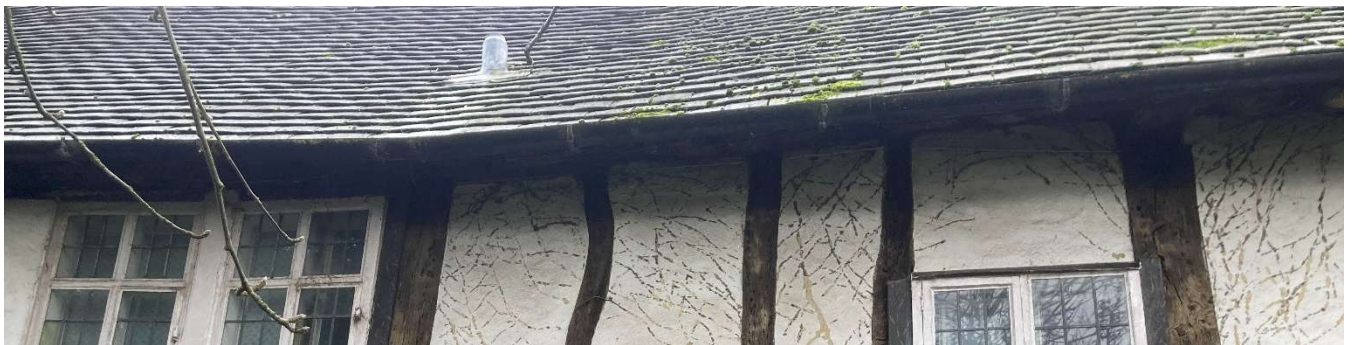
Possible gutter deformity creating leaks
