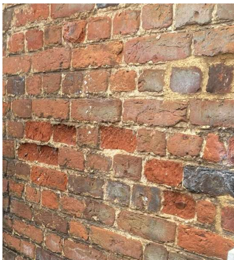
Brick face erosion and signs of 'Penny Roll' pointing
