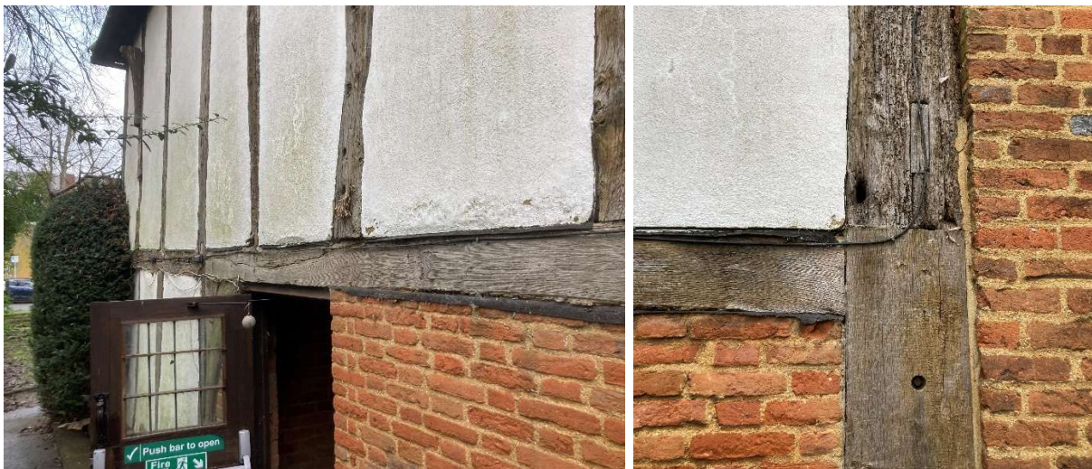
'Hollow' sounding replacement oak and decayed stud bases Note the roof felt flashing detail used both top and bottom here.
