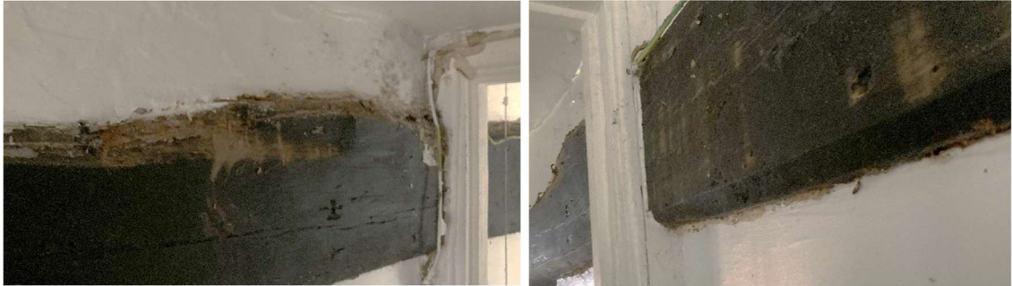
Slight decay in the top and bottom of a principal beam in Flat 6
