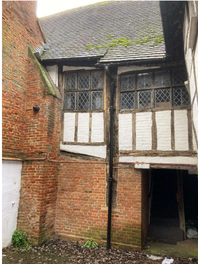
Damp in the north facing elevation within the courtyard
