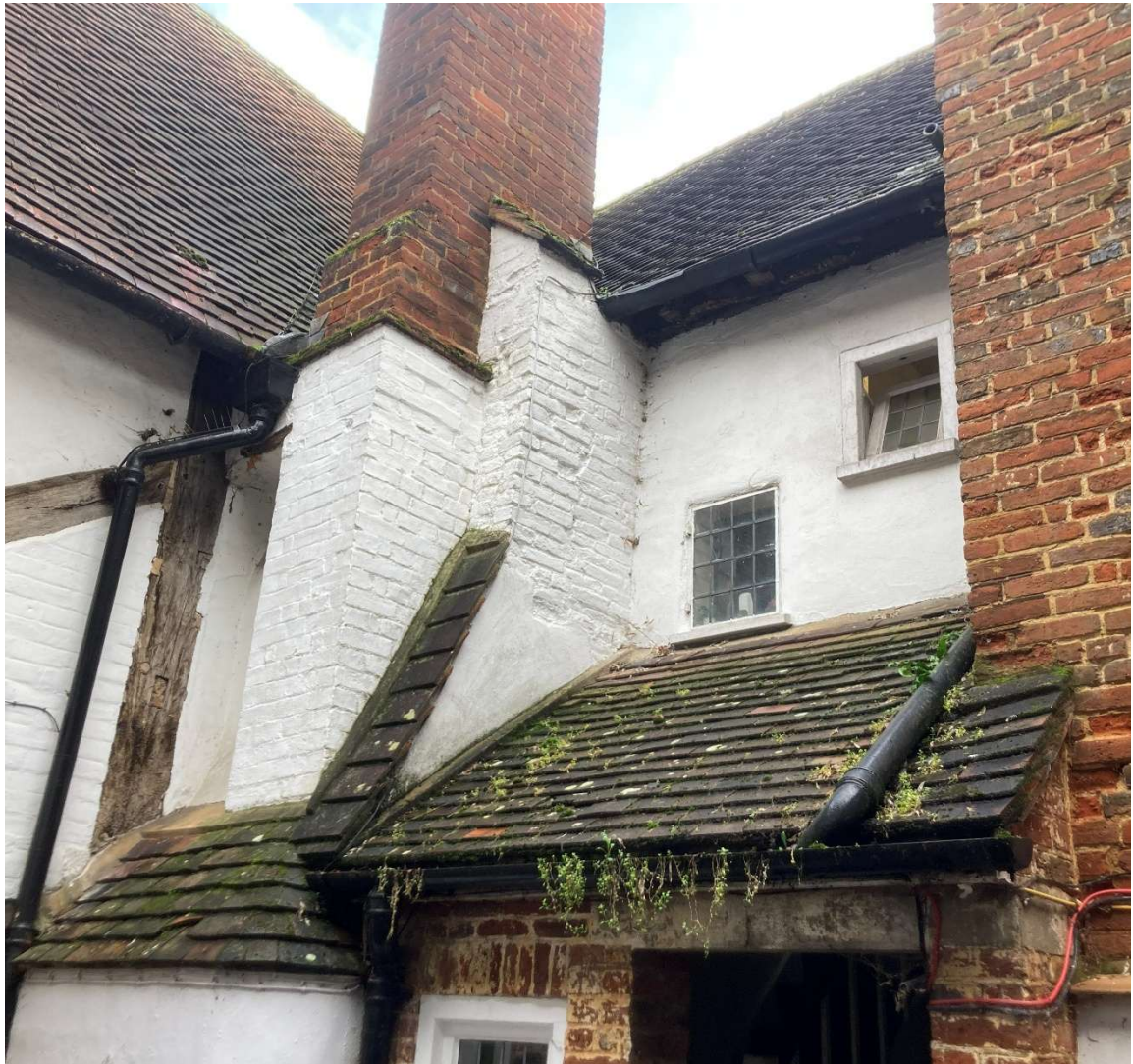
South-west facing corner with damp and vegetation on tiled slopes
