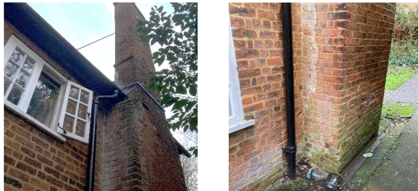
Efflorescence along side of chimney – probably due to historical failure of the gutter and downpipe
