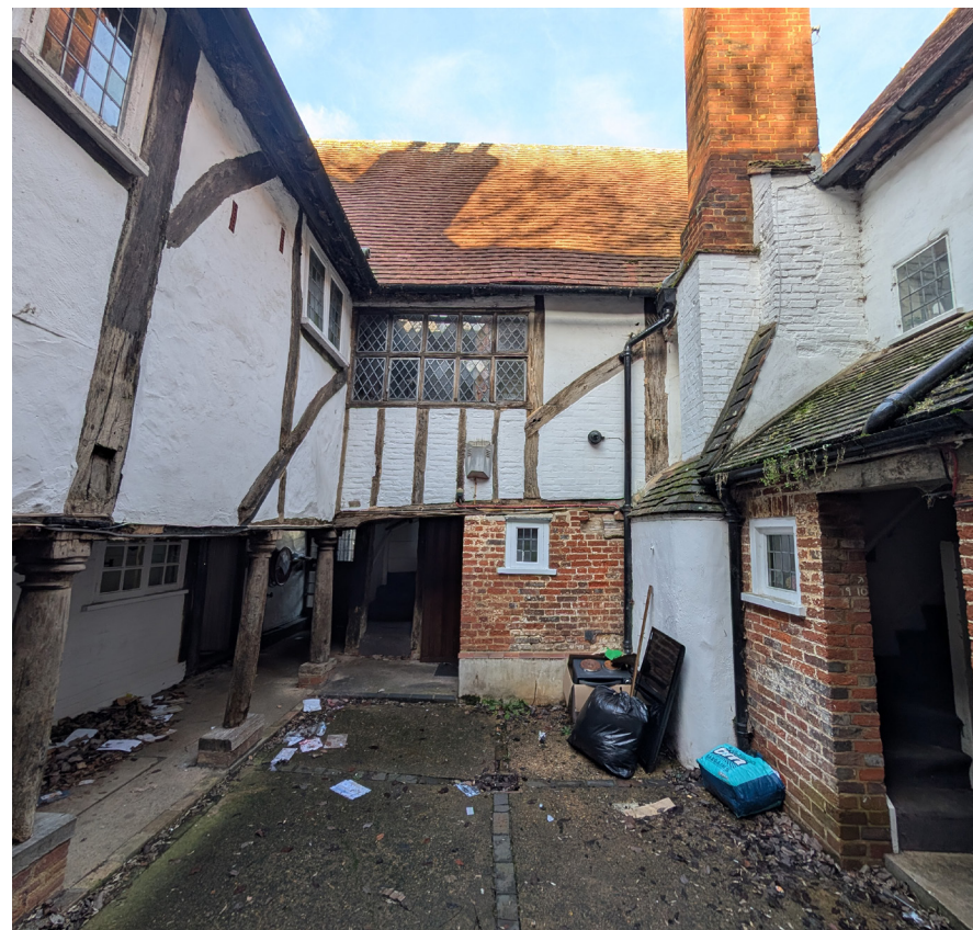
Existing Courtyard in very poor condition, damp and littered
