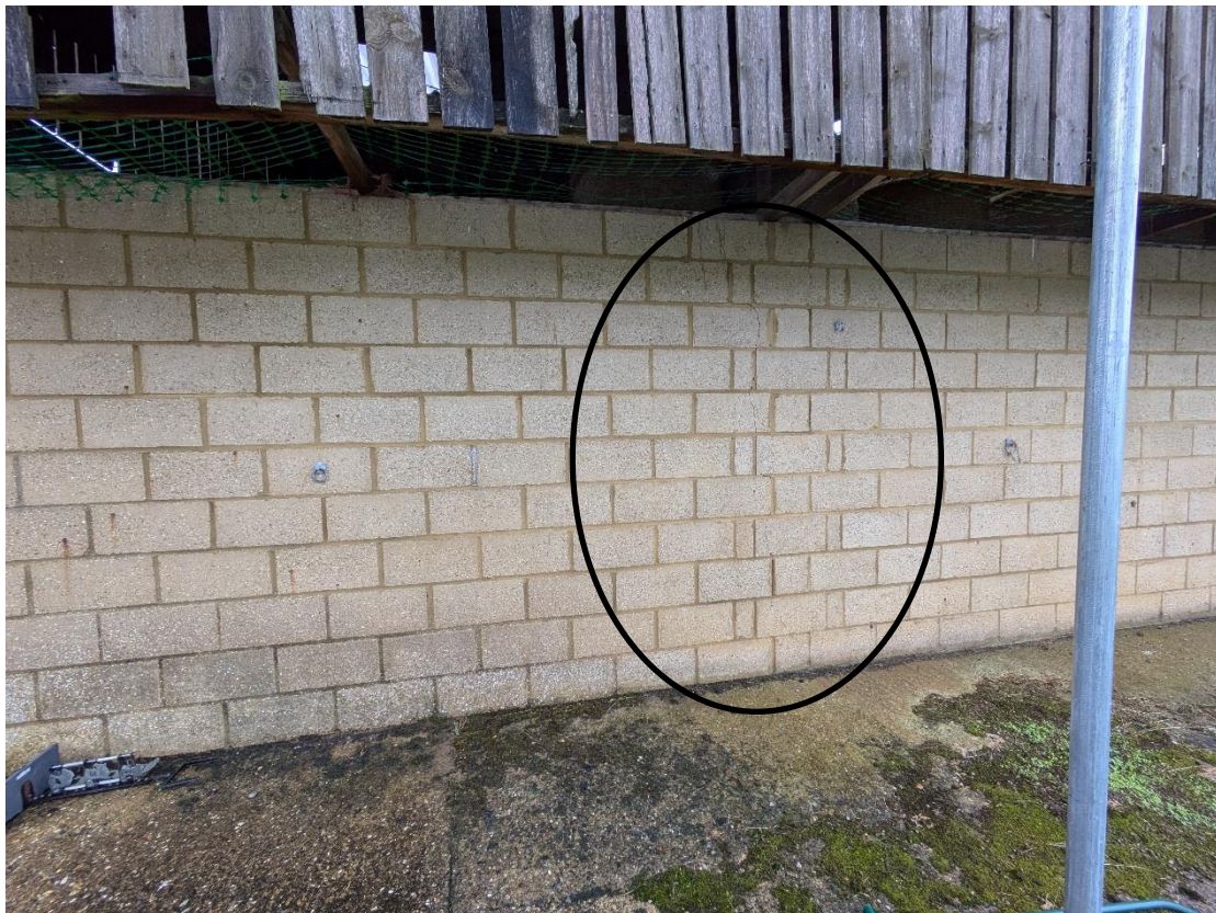
Photograph 7 Left hand side elevation – typical vertical hairline crack.
