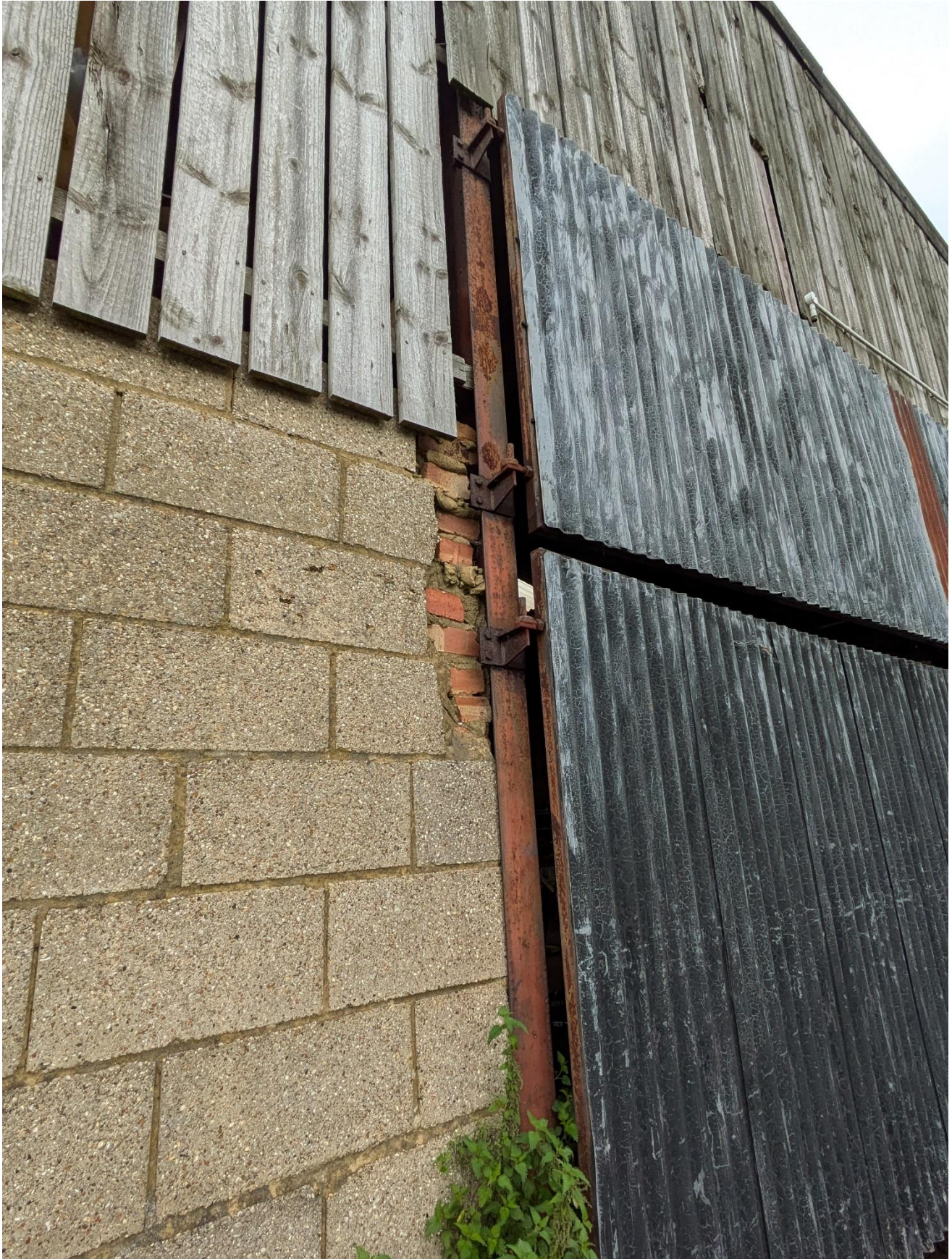
Photograph 8 Typical views on loss of mortar at doors.
