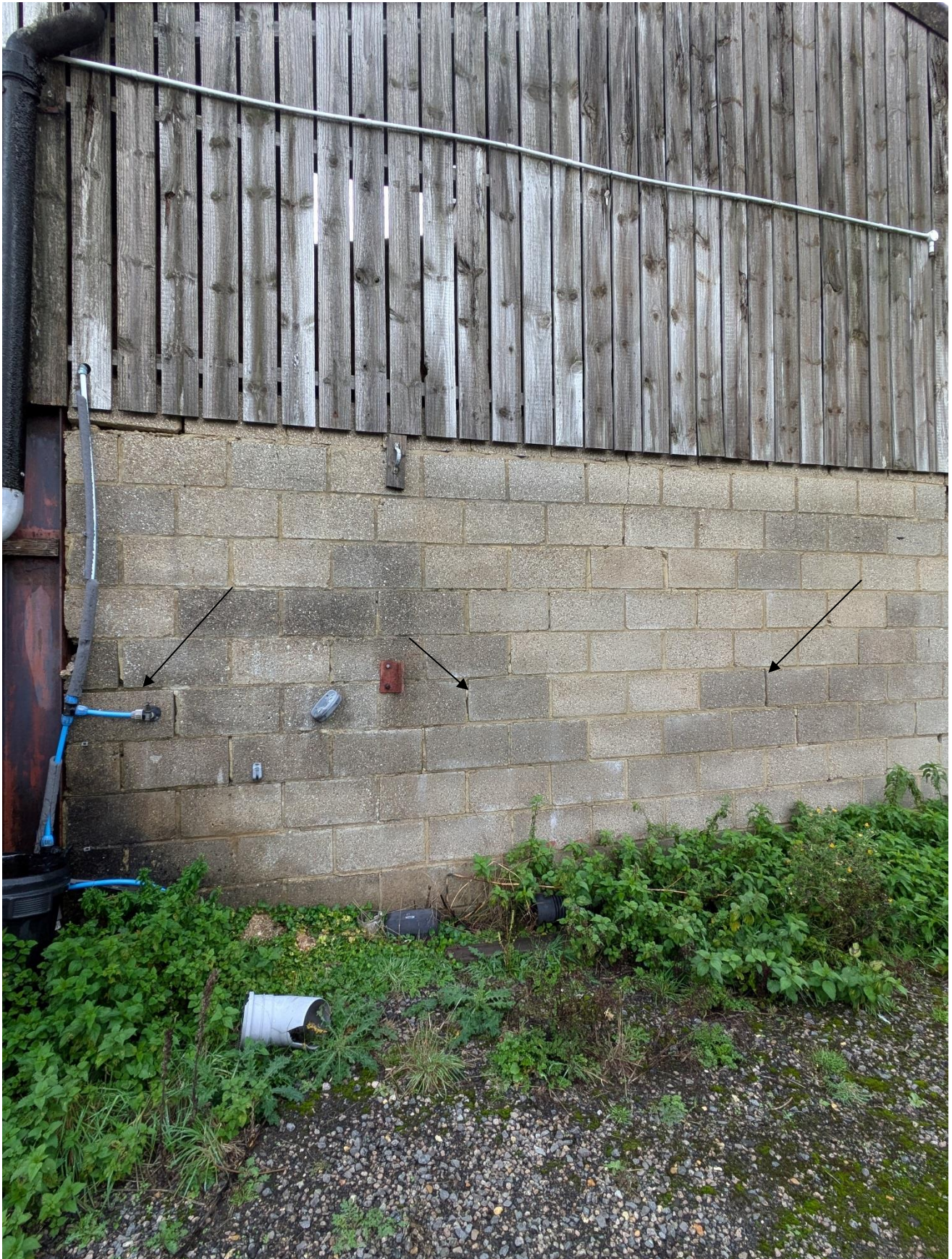
Photograph 9 Rear elevation – cracking in bay to right hand side of water butt.
