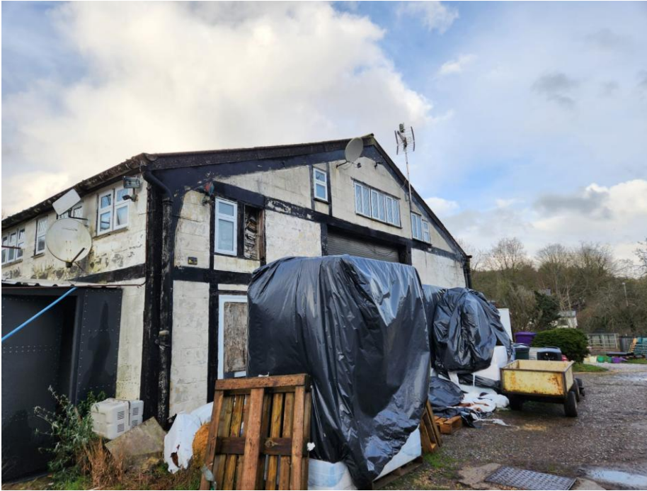
Plate B.1 Main farm building on-site (B1), showing mixed construction and potential features suitable for bats.
