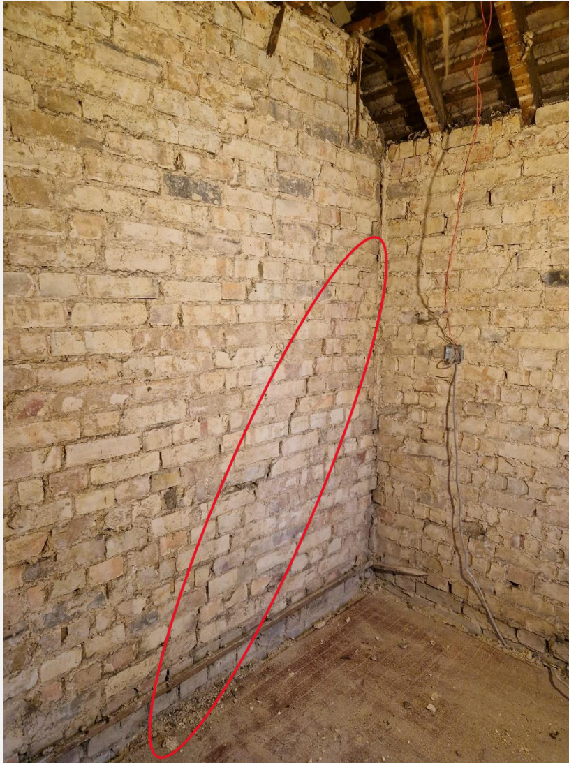
Figure B – Stepped cracking in the front room nearest T013
