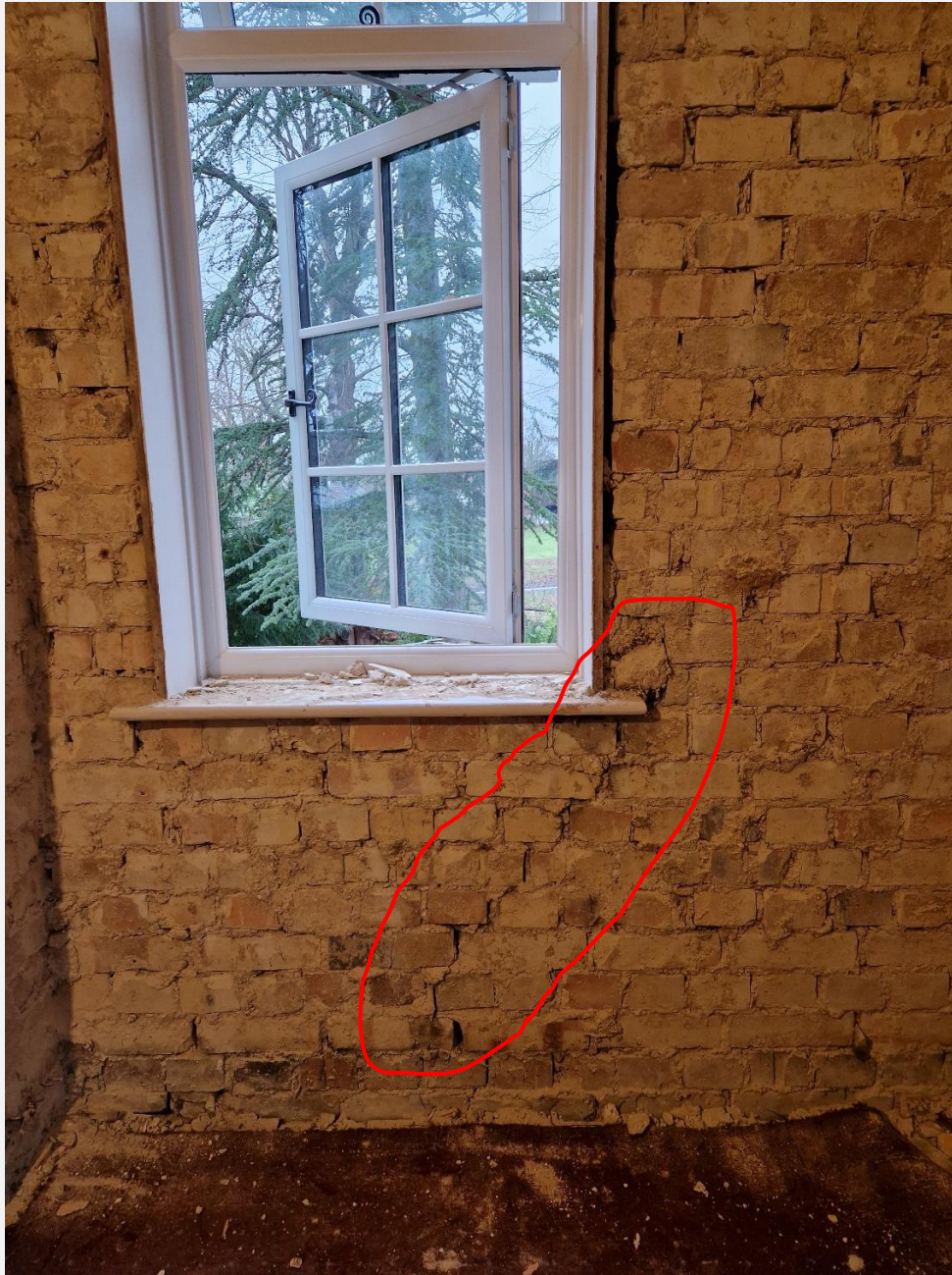
Figure A – stepped crack in the wall with offending Cedar in the background
