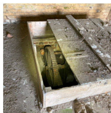
The well in the Tank House
