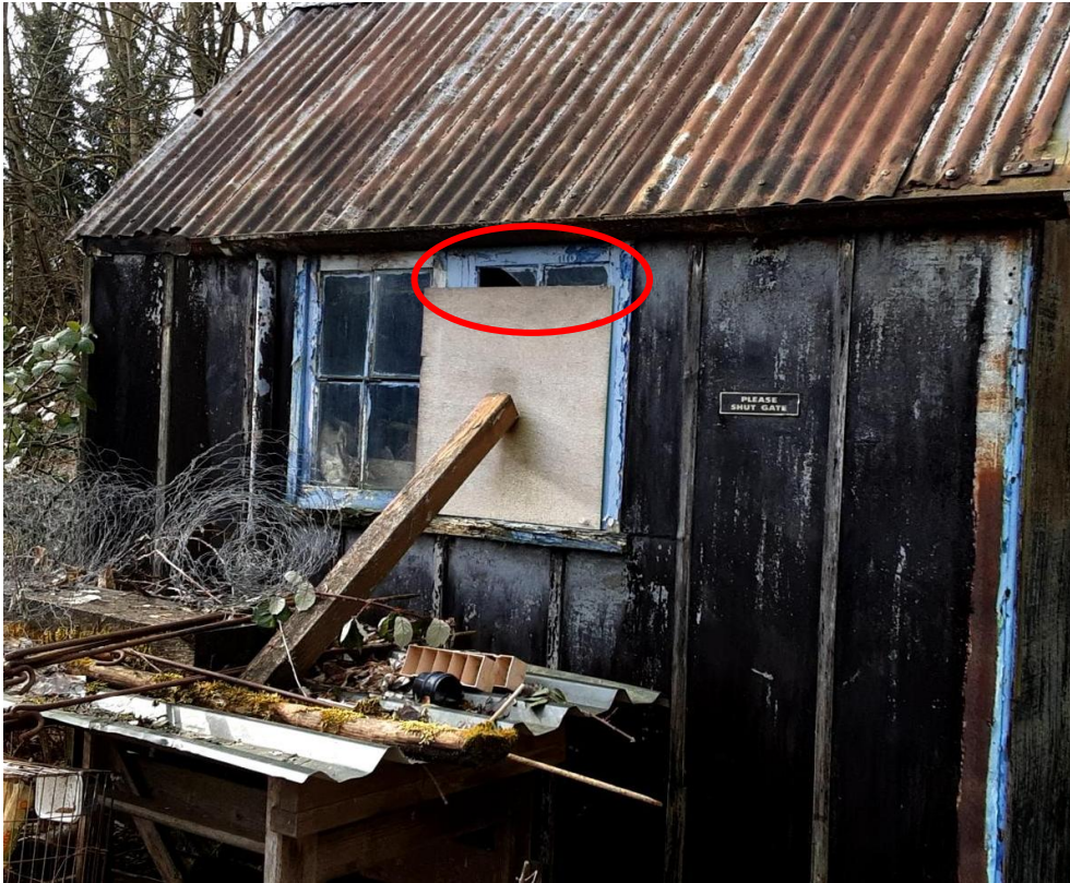
Photograph 4: Building 2, broken window on eastern aspect
