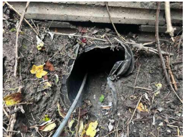
HW4 Outfall deformed
