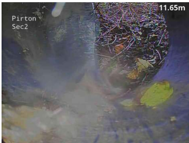
5, 00:01:39, 11.80 m Deformed sewer or drain, 40%
