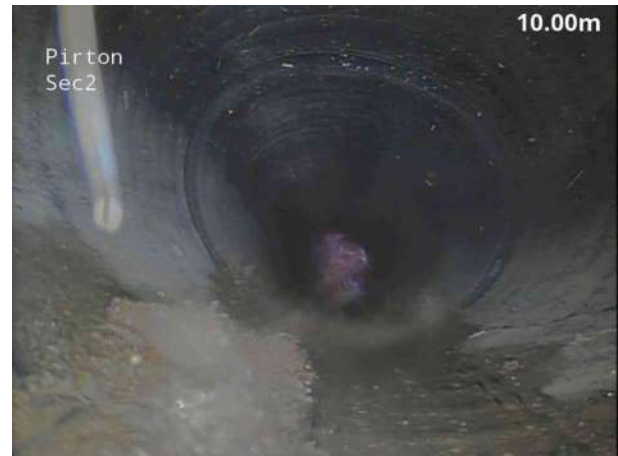
4, 00:02:08, 10.20 m Deformed sewer or drain, 15%
