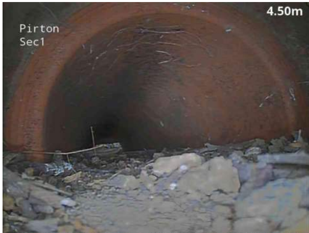
7, 00:01:22, 4.50 m Pipe material changes to vitrified clay at this point
