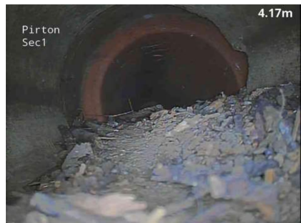
6, 00:01:22, 4.50 m Pipe material changes to vitrified clay at this point
