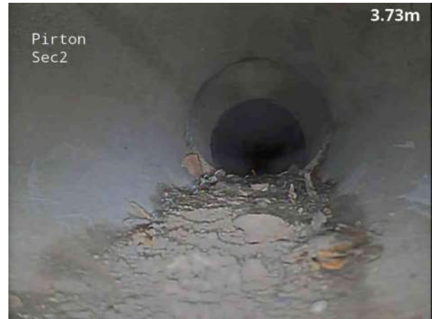
2, 00:00:35, 4.00 m Settled deposits, coarse, 10% cross-sectional area loss
