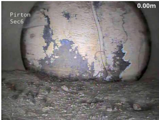
1, 00:00:00, 0.00 m Settled deposits, fine, 10% cross-sectional area loss
