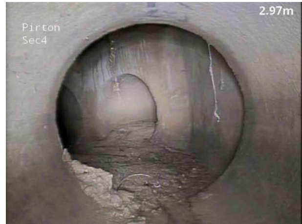
2, 00:00:25, 3.20 m Settled deposits, fine, 10% cross-sectional area loss, finish
