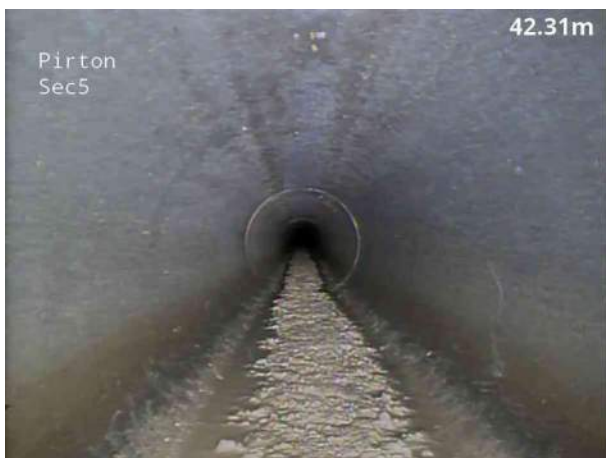
3, 00:04:38, 42.30 m Survey abandoned, Unable to continue, assumed cable drag
