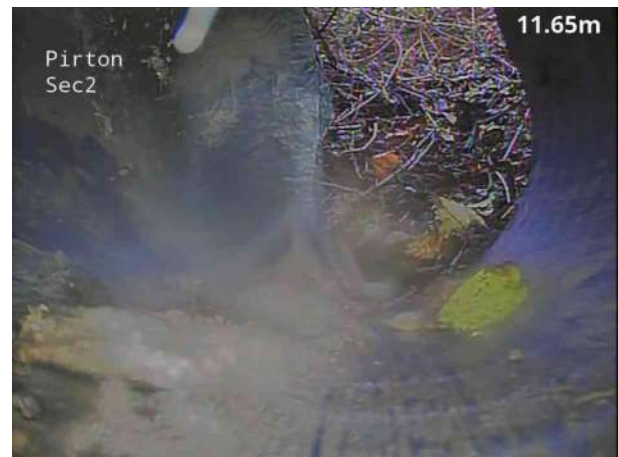
6, 00:01:39, 11.80 m Deformed sewer or drain, 40%
