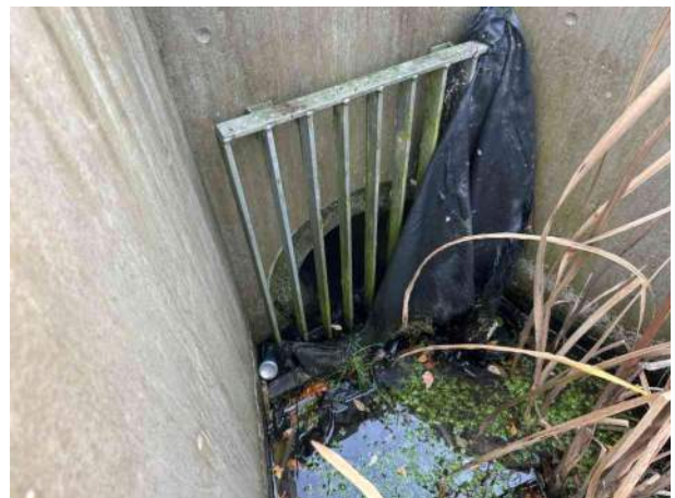
375mm Outfall from balancing pond
