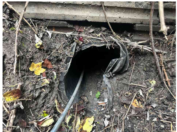
HW4 Outfall deformed
