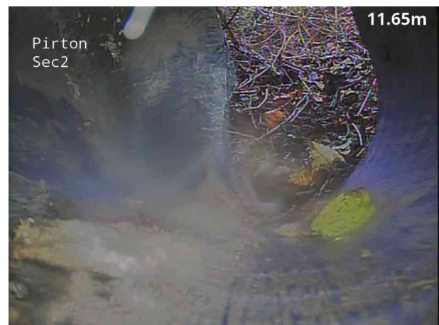
6, 00:01:39, 11.80 m Deformed sewer or drain, 40%
