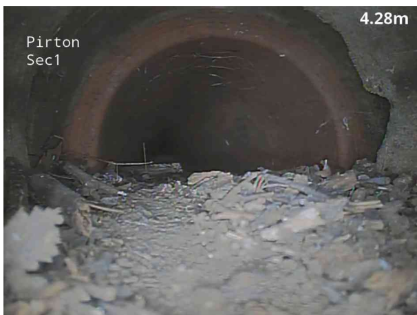
5, 00:01:19, 4.50 m Hole in drain or sewer from 9 o'clock to 3 o'clock
