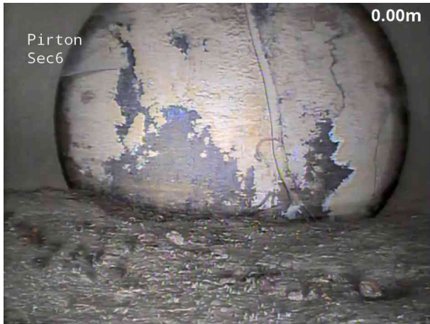
1, 00:00:00, 0.00 m Settled deposits, fine, 10% cross-sectional area loss
