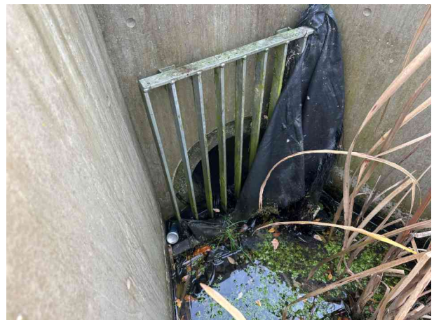
375mm Outfall from balancing pond
