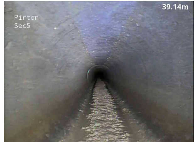
2, 00:03:15, 39.00 m Settled deposits, fine, 5% cross-sectional area loss, change
