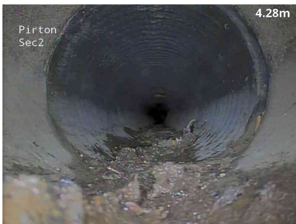
3, 00:00:47, 4.50 m Pipe material changes to polyvinyl chloride at this point
