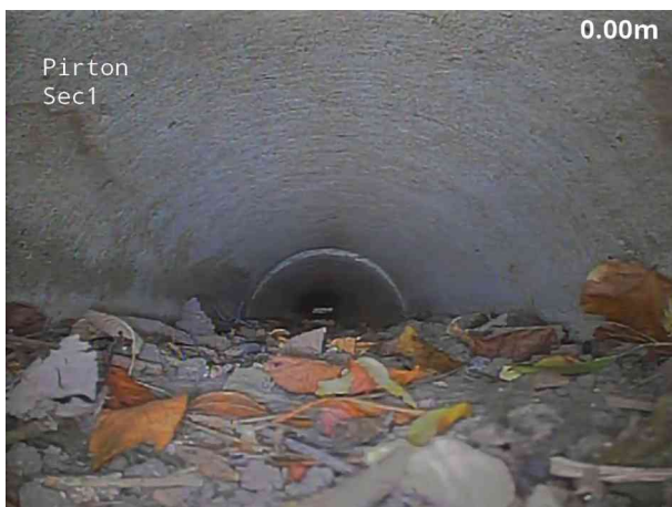
3, 00:00:25, 0.00 m Settled deposits, fine, 40% cross-sectional area loss, start
