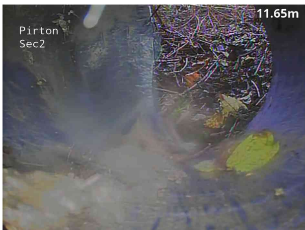
5, 00:01:39, 11.80 m Deformed sewer or drain, 40%
