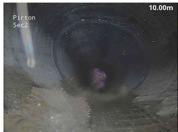
4, 00:02:08, 10.20 m Deformed sewer or drain, 15%
