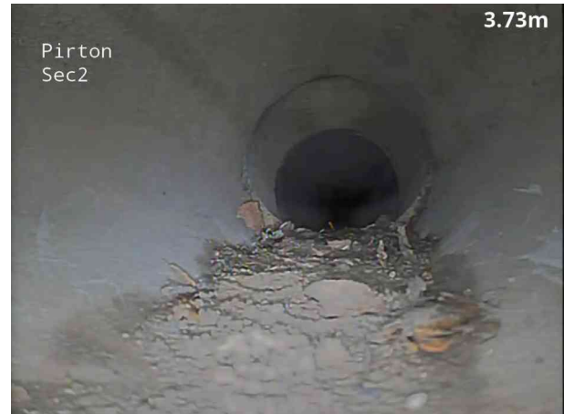
2, 00:00:35, 4.00 m Settled deposits, coarse, 10% cross-sectional area loss
