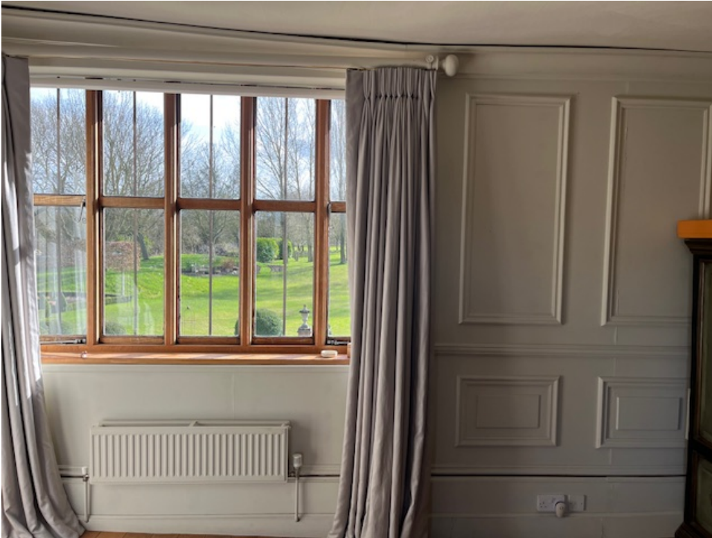
Photo 7.1 - modern wall panelling to be removed.
