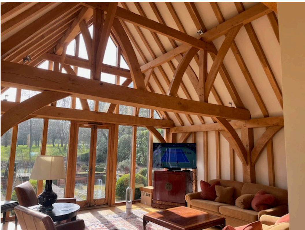
Photo 5.2 - redundant non-structural oak brackets to be removed.
