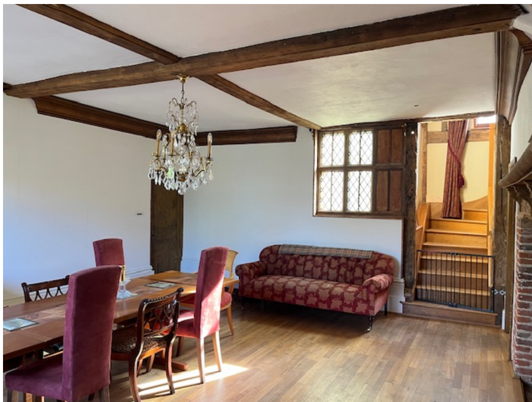
Photo 2.1 - modern cornice and modern skirting to be removed.
