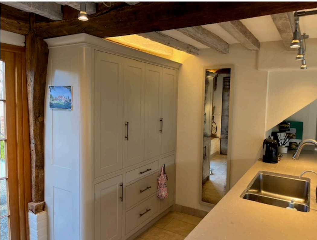
Photo 4.2 - modern cabinets to be removed.
