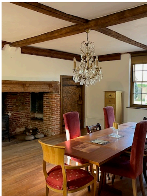
Photo 2.2 - modern cornice and modern skirting to be removed.
