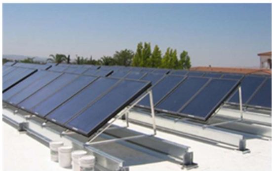
Figure 7.3—Frame mounted PV on flat roof
