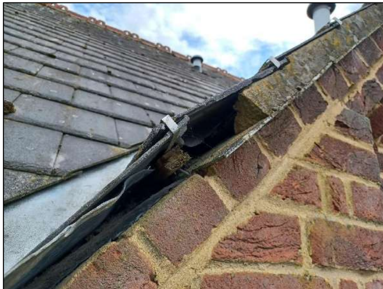
Photo 7: Example damage to roof, suitable for roosting bats.
