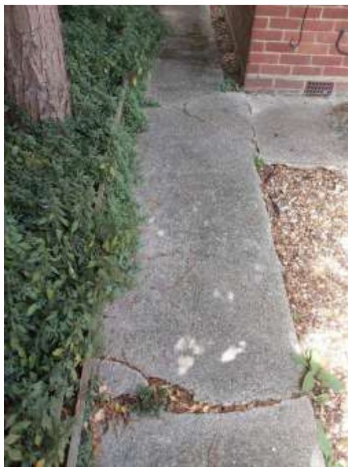
Plate 2: Direct damage caused by secondary root expansion of T001.
