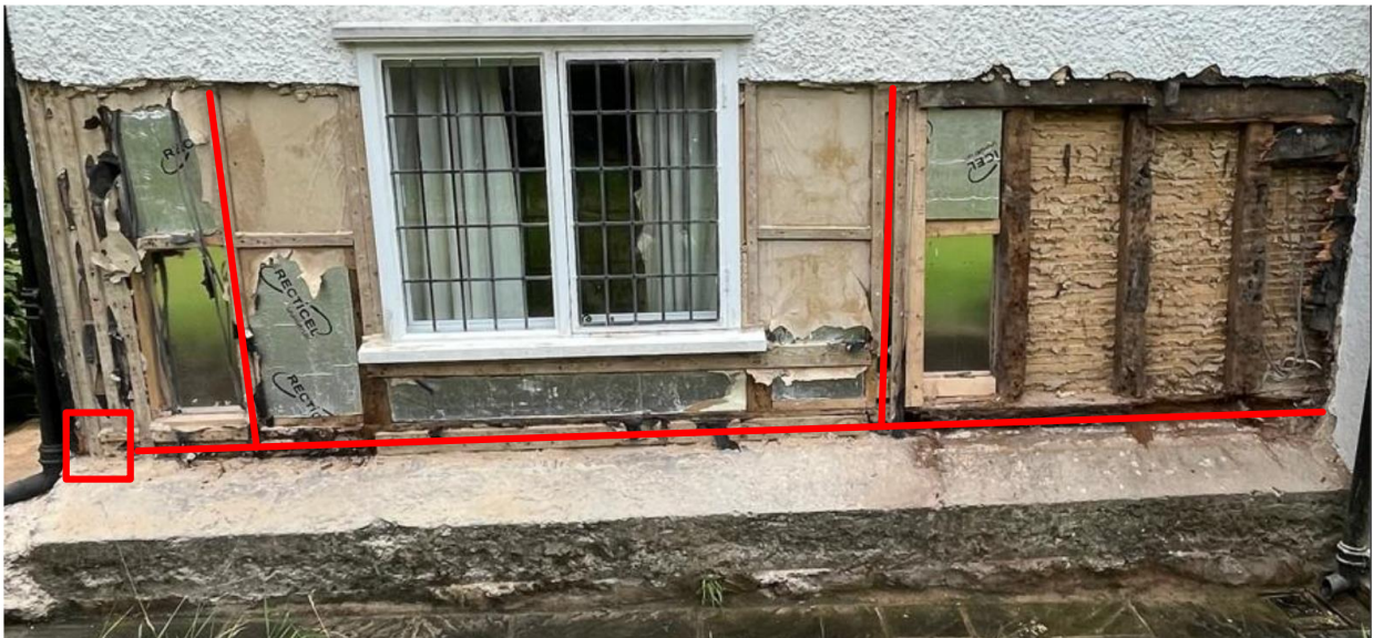
Figure 3: North Elevation with Render removed approximately 1.2m from sole plate
