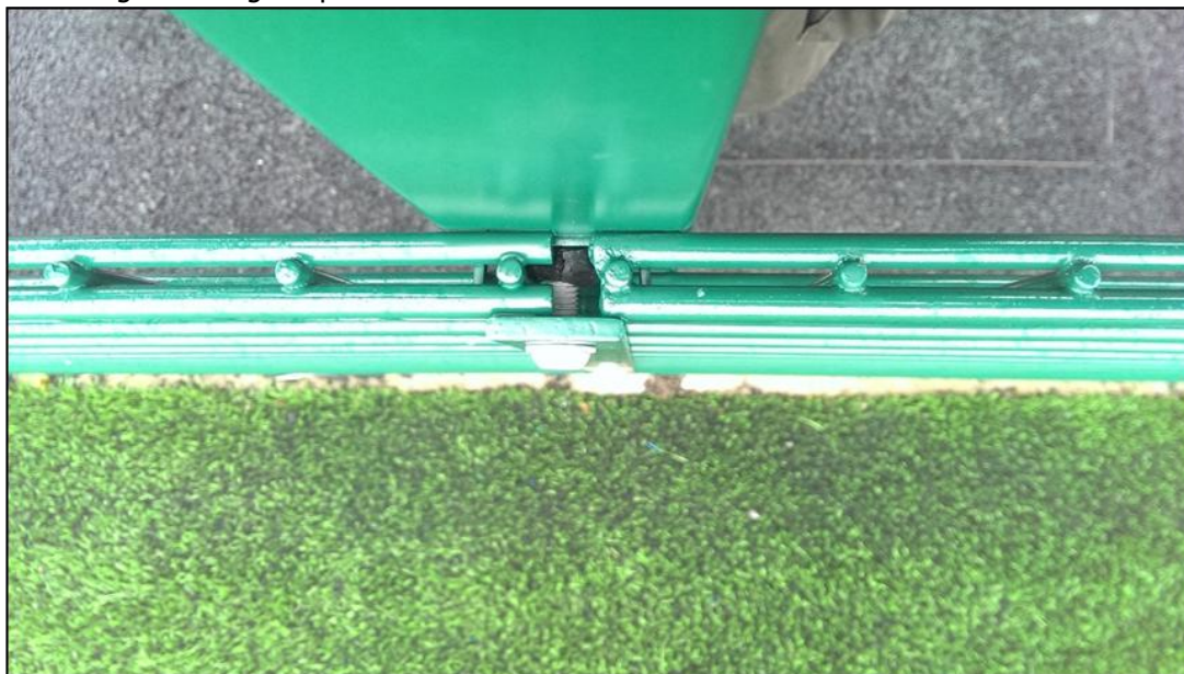
Figure 8: Image showing neoprene isolators
