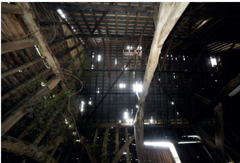
PHOTOGRAPH SHOWING FAILURE OF ROOF COVERING AND EXTERNAL CLADDING OF LISTED BARN
