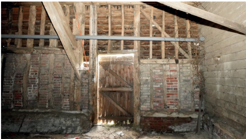
PLINTH & FRAMING TO BAYS J & K IS INCONSISTENT
