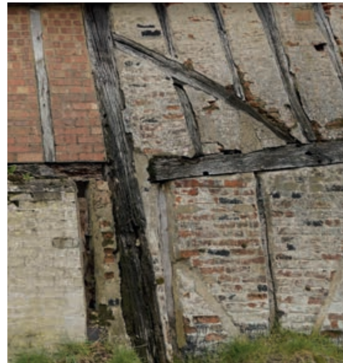
EXAMPLE OF SERIOUS DECAY TO TIMBER FRAME OF WEST ELEVATION OF BARN TWO
