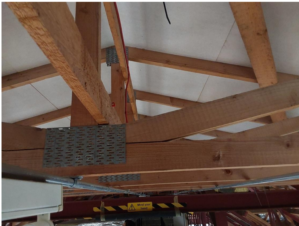
Photograph 15: Example of gaps present between wooden support beams
