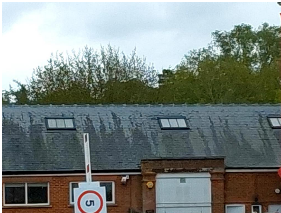
Photograph 10: TN6 – Lifted flashing around windows
