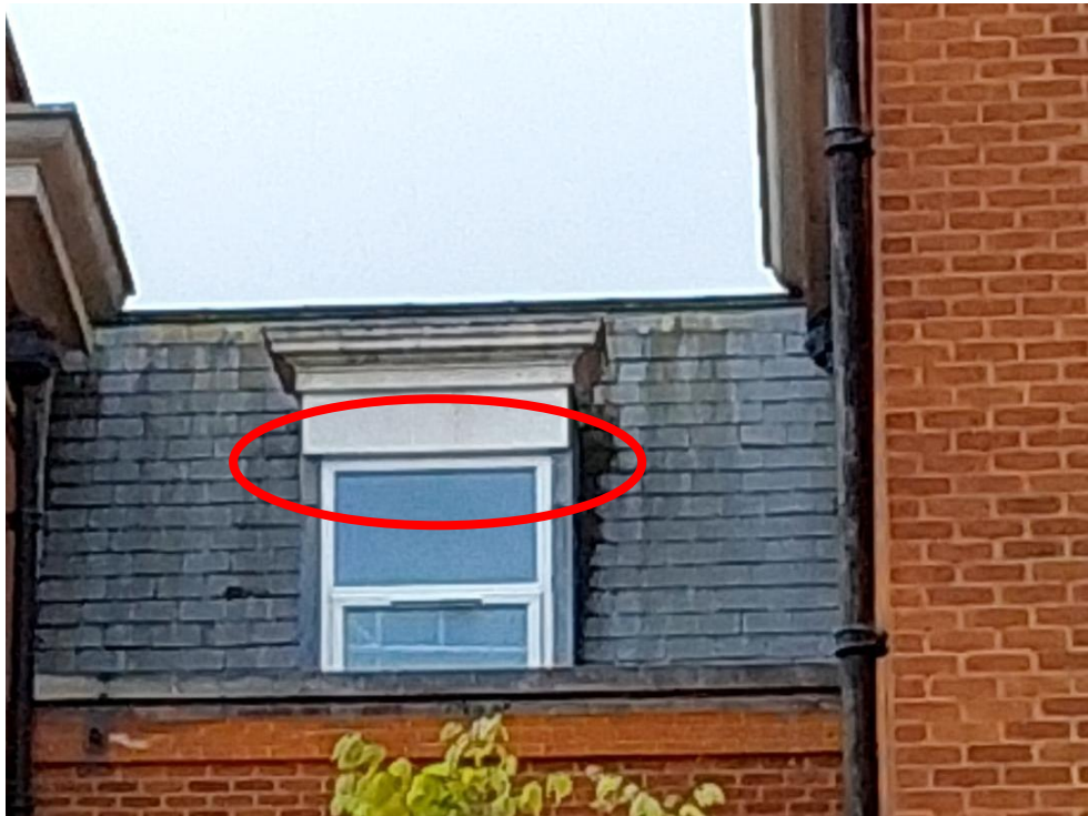
Photograph 9: TN5 – Gap between board and flashing on dormer window
