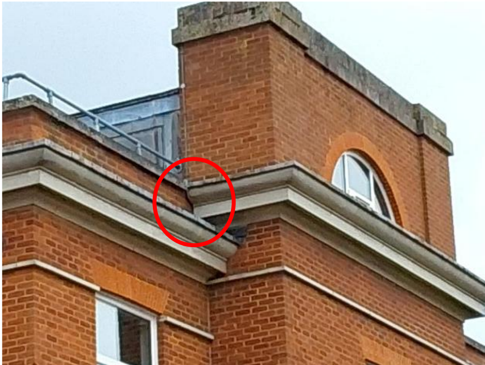
Photograph 11: TN8 – Gap between concrete and brick wall
