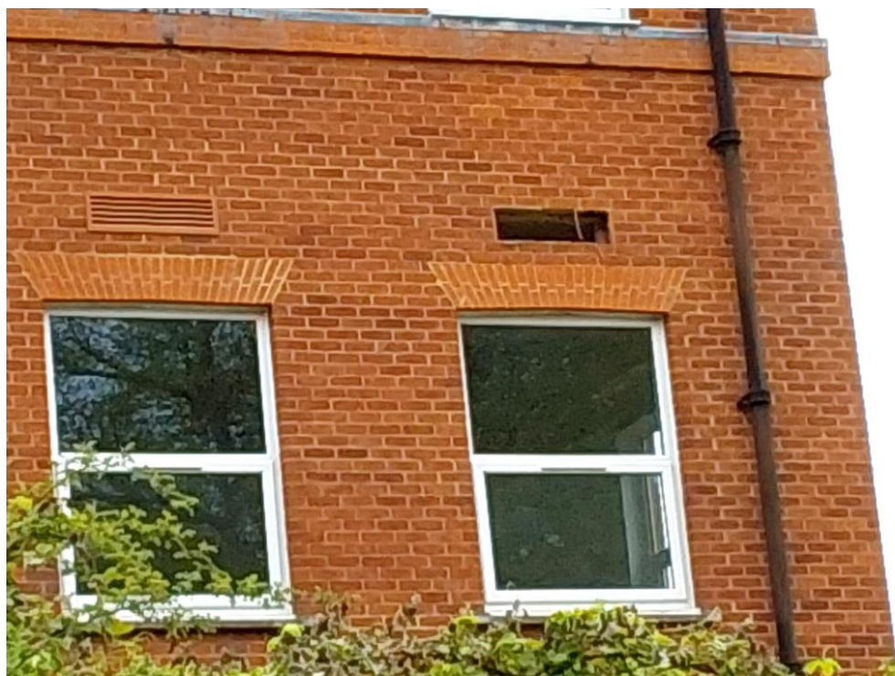
Photograph 8: TN2 – Large cavity where a vent cover is missing
