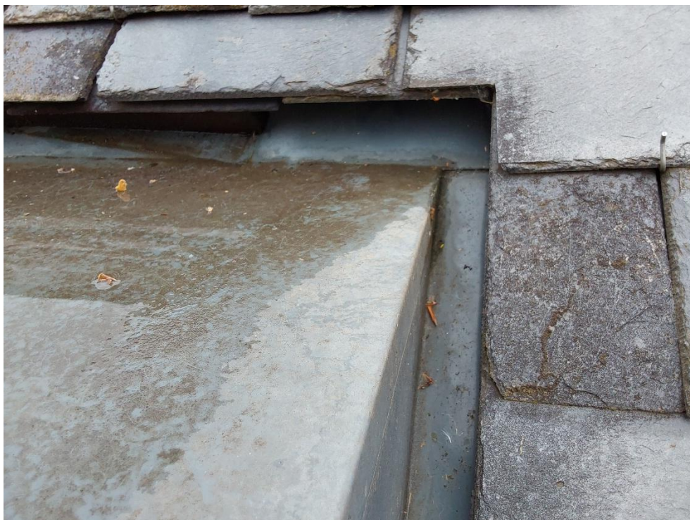
Photograph 12: TN9 – Gap under the tiles where a wooden board has dropped
