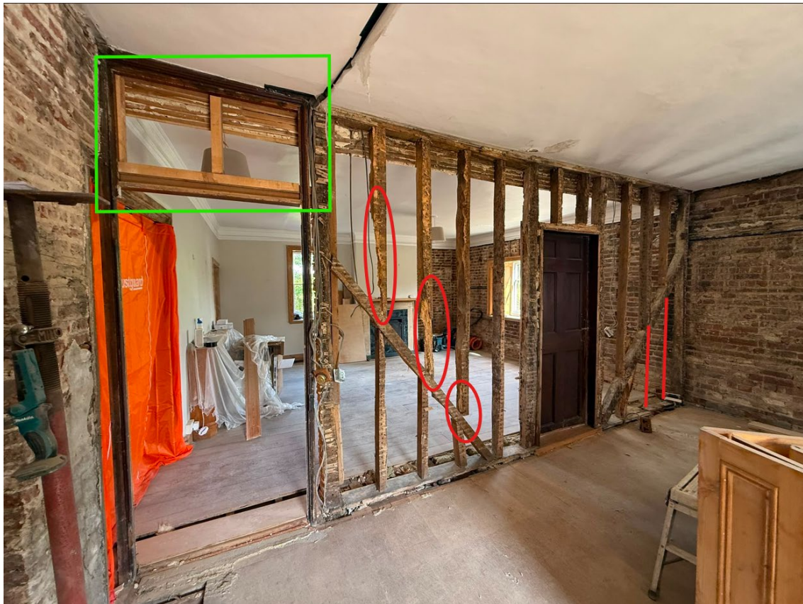
East wall of Living Room: Green denotes C21st fabric; red shows missing or badly damaged studs. Note that the 'soleplate' is a board resting on brick infill to the ceiling joists of the basement below.
