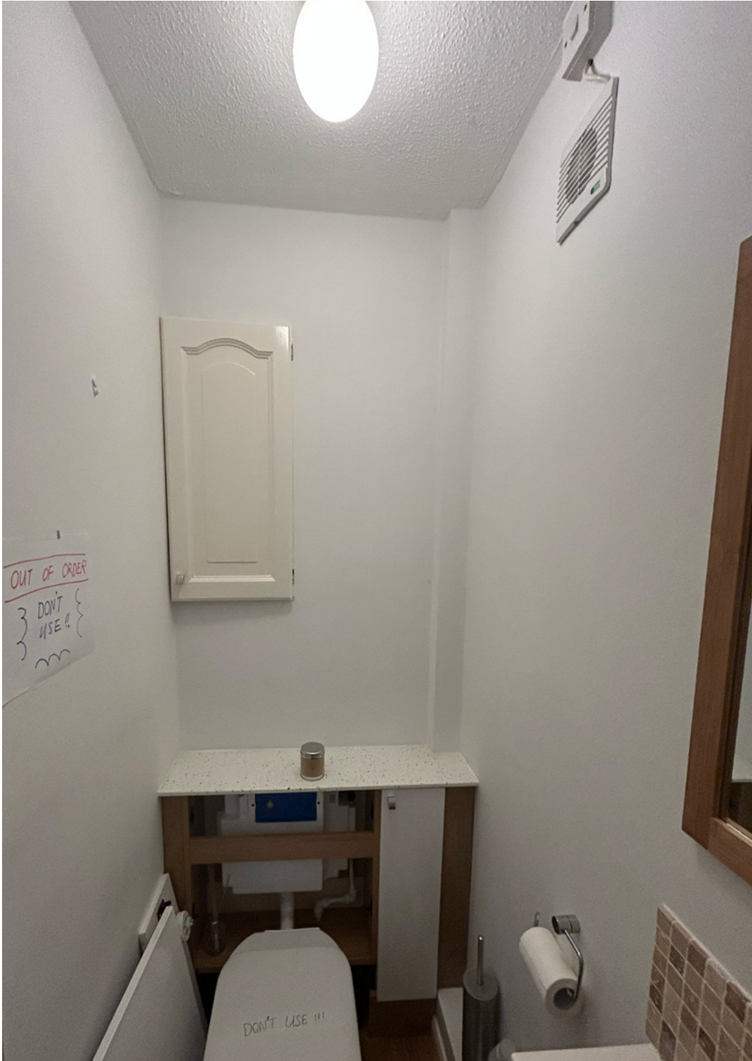
Ground Floor Toilet out of order
