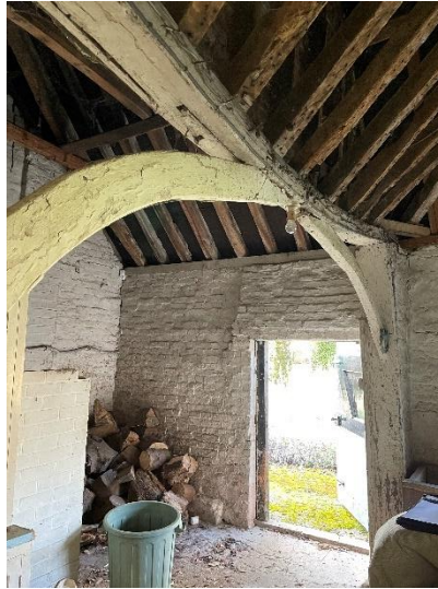
Timber brace to be repaired/strengthened
