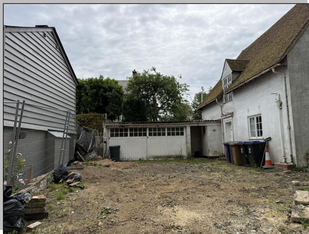
Photograph indicating the existing garage/workshop/potting shed to be demolished, and its relationship with the neighbouring property 'Hodwell Barn' to the east. A brick boundary wall between the two properties is to be rebuilt after its collapse.
