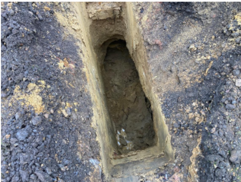
TP2 – collapsing sides and running sand
