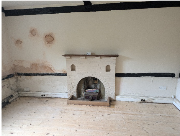
Walls showing damp in front room, fireplace non original
