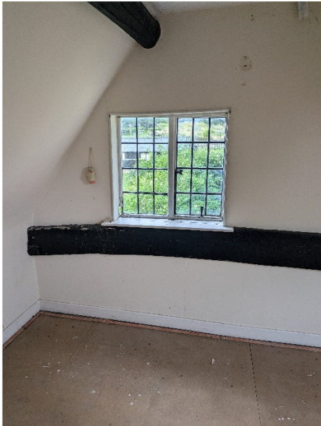
Window frame to be replaced & sashes reused. W14
