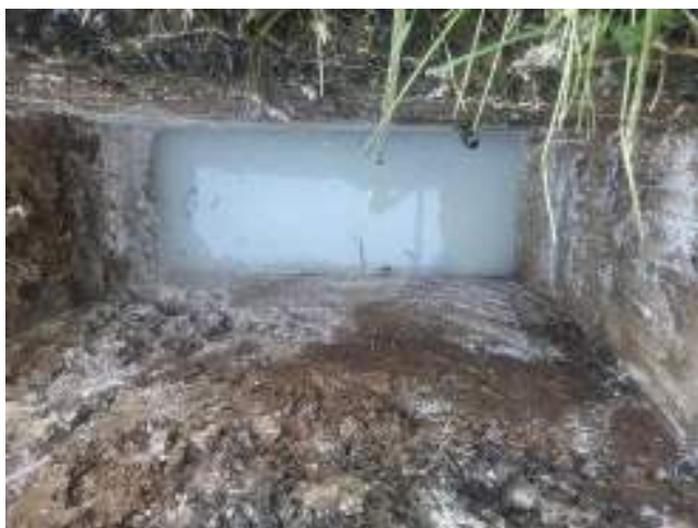
Photo 2: TP1 filled with water
